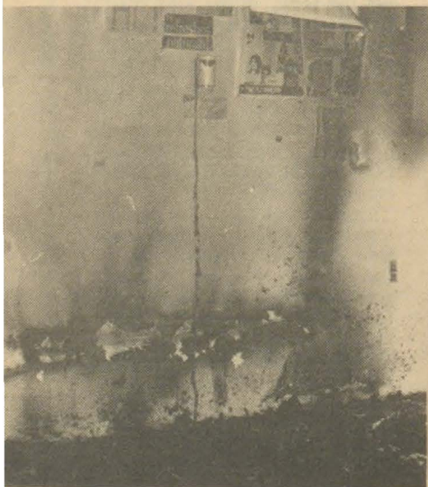
The fire was started by a faulty electrical cord running along the north wall.
